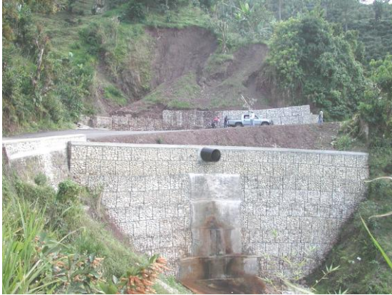
Figure 4. Elaborate gabion works installed at Spring Hill, Buff Bay River valley. Landslide (background) had obliterated the road. The source area still having portions of the slipped mass is clearly visible. This structure is a combination of step-gabion baskets and mattress gabion baskets (partially seen at base of photograph). Note the large drainage pipe at the centre of the photo. Poor drainage is a major trigger of slope failures throughout Portland. Remediation measures such as this are quite costly [R. Green, Feb. 2007]
