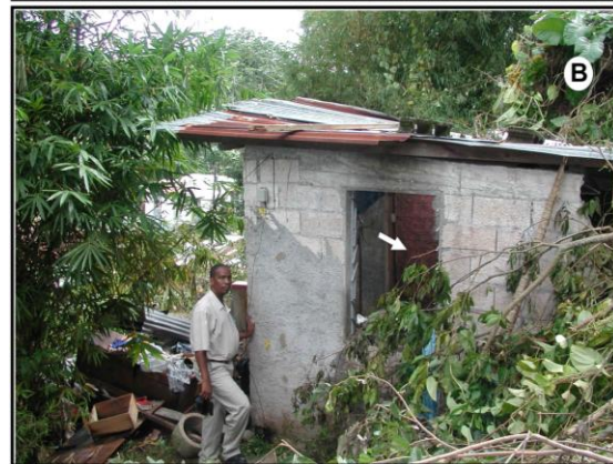
Figure 2. Rainfall-induced landslide at 4 Red Hassle Road between Port Antonio and Breastworks. Rainfall period Nov. 19 – 25, 2006. A: View from main road at base of landslide; note that the house has been obliterated with the landslide debris. B: Side view of destroyed house. The body of a woman that died was dug from the doorway of this partially intact bedroom (marked by arrow). [R. Green, Nov. 30, 2006].
