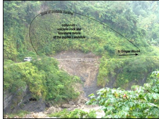
Figure 5. Landslide at Friday, south of Ginger House, Rio Grande valley. Landslide (centre) has reduced the road to narrow single lane. The landslide is very active, continually retreating over the last 10 years. It continues to fail as the unstable colluvial material slips from the steep slope above in the zone of unstable material delineated by secondary shrubbery. Colluvium consists of debris of volcanic rock and limestone originating from across the river (behind photographer). Note that the colluvium overlies the shale which shows distinct bedding in the river bank (lower left-hand corner). Beds dip towards the river encouraging planar failure in the colluvium. This particular landslide has made several news reports as the locality is hazardous to road users. The latest was 2009 when a vehicle toppled over and became lodged just below the roadway. [S. Bhalai, June 2009]
