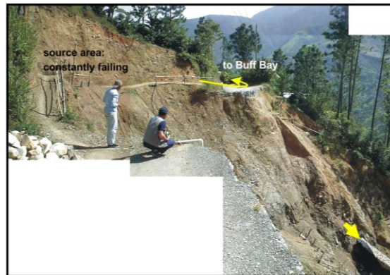
Figure 3. Composite showing break-away at Section, Newcastle to Buff Bay main road. The source area of the landslide is continually retreating, constantly destroying the footpath cut on the left. At the extreme bottom-right-hand corner of the plate is the remediation gabion works under construction (thick arrow). Informal communication with resident in 2006 revealed that this installation will cost $3 million. [S Bhalai, Aug. 2006]
