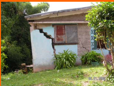
Earthquake damage - June 12, 2005,.
